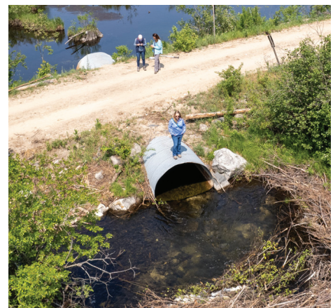
Program Director Kim Balke shows C3 team members an undersized and ecologically damaging culvert on Jordan River Road.
