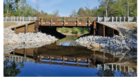
The new Douglas Lake Rd. crossing serves as a finish line for the now freed Maple River.
