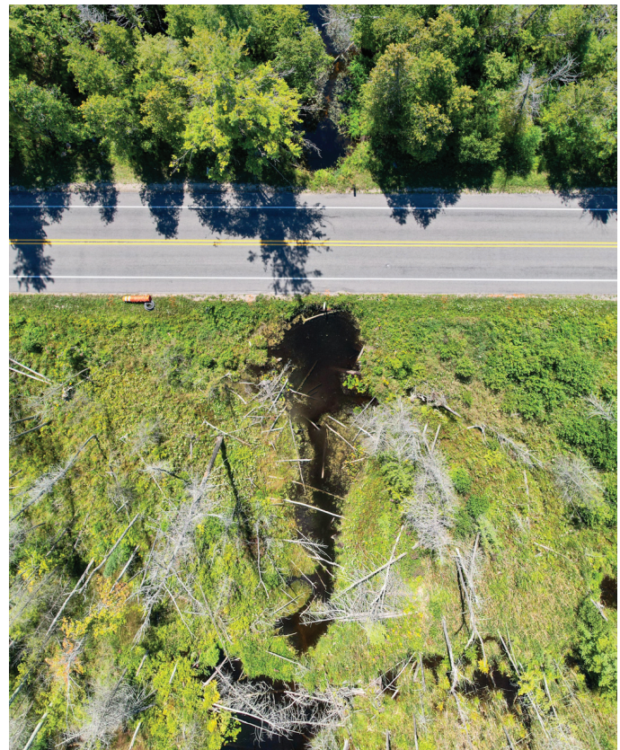
At the Tucker Lake Outlet, a blocked and severely undersized culvert results in water pooling on both sides of Leelanau County Road 675, increasing the risk of road flooding.
