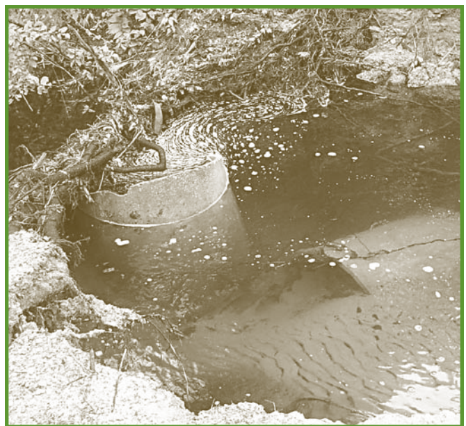
Inadequate road crossings can lead to failure in extreme rain events. Tons of sand dumped into a stream takes years and years to wash out of the system. The rains this June washed out over 60 crossings in Northern Michigan.
