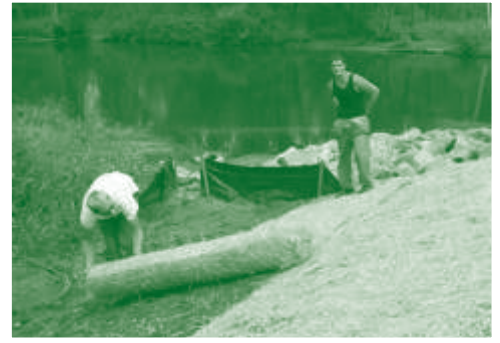
Subcontractors roll out straw mulch matting to help revegetate the embankments at Indian Bridge.
