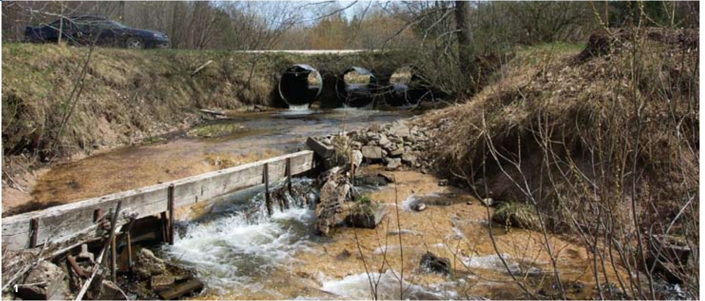
1. Before - aging culverts and dam remnants were an unsightly problem on Dair Creek. 2. After - a bottomless arch accommodates fish passage.
