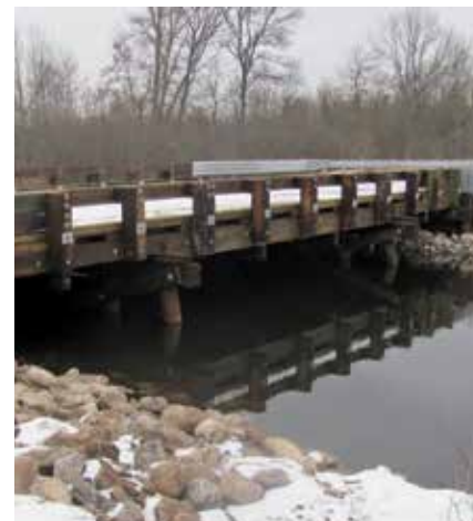
The new channel spanning timber structure allows for unrestricted aquatic species passage and sediment and nutrient movement.
