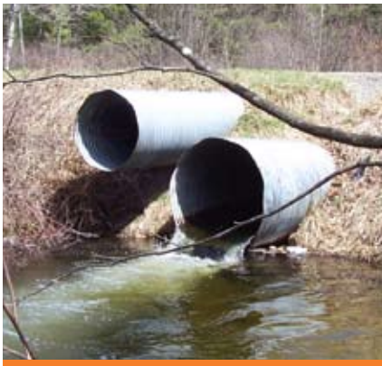
Perched culverts prevented upstream fish passage.
