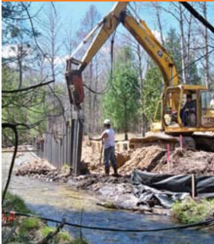
The McDowell Construction crew drive sheet piling for the new crossing structure.
